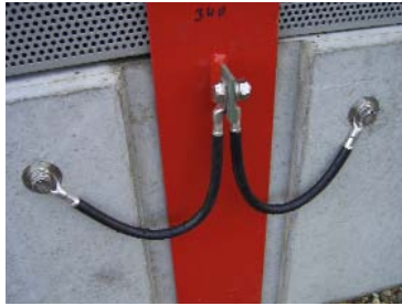
earthing terminals at base elements
